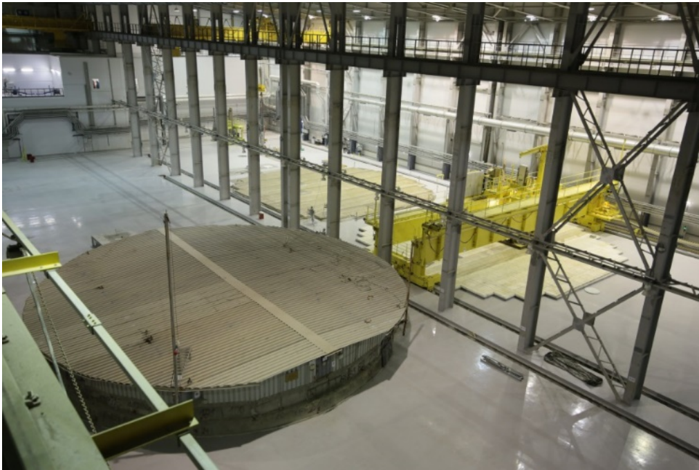
Figure 6. General view of the storage tanks at the DSU-3A in Building 153.
