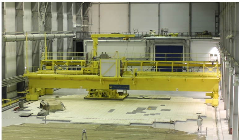
Figure 5. Handling machine above the DSU-2A tank.
