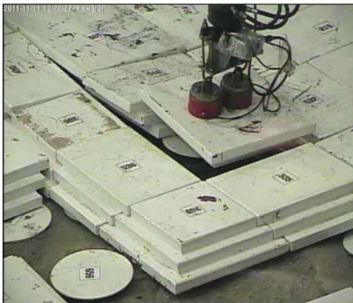
Figure 3. Installation of the biological shielding on the surface of the DSU-3A tank.
